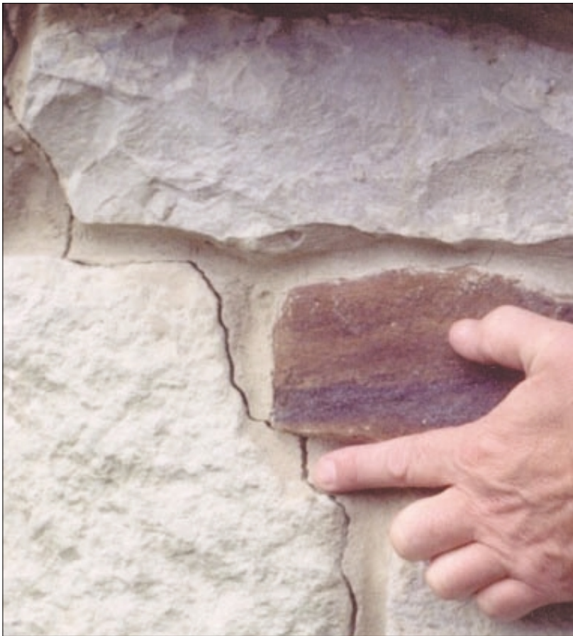
Fig 13. (left) This crack is aesthetic damage only
