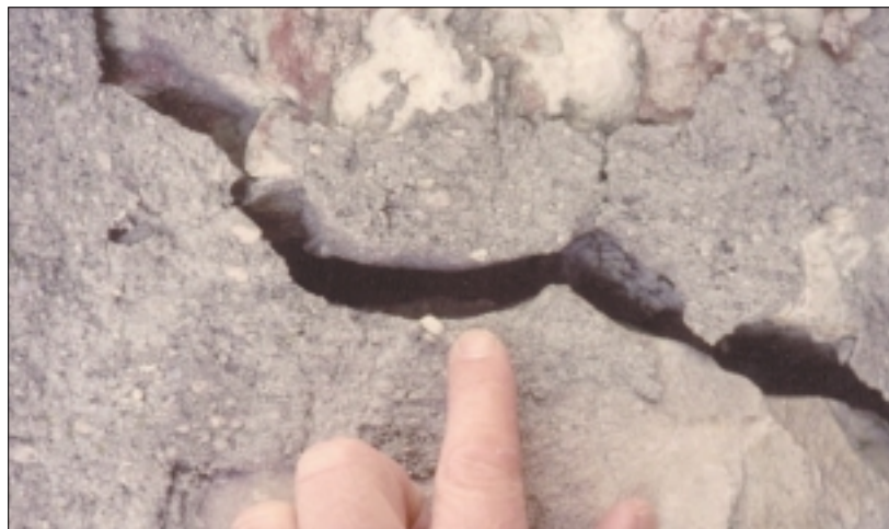
Fig 2. This crack has probably been filled before, with cement mortar. The wall appears to be random stone wall laid originally in lime mortar. The repairs to part of it with cement mortar can alter the manner in which it behaves
