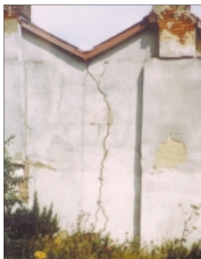
Fig 1. Is that crack serious?
