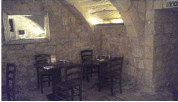
Figure 5: this basement construction in Rabat probably pre-dates the overlying 16 th century palatial construction. Rubble infill masonry abuts onto the street walling, whilst the supporting masonry arch quoins are formed in ashlar masonry. 1m masonry slabs span onto the arches, whilst flooring is in tal-qawwi flagstones. (SOURCE: Author)
